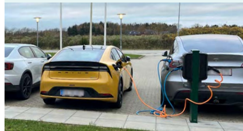
Charging points for electric and hybrid cars at Gibo Plast A/S.
